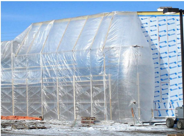
Typical Temp Enclosure
